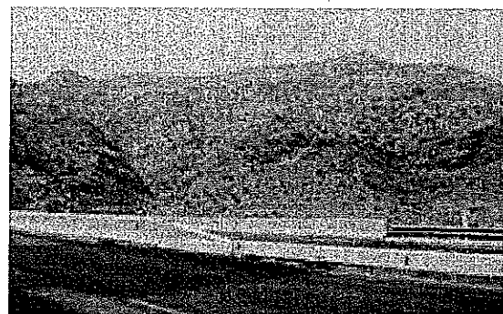
Settlement of Bridge Approach (Bridge No.4)
